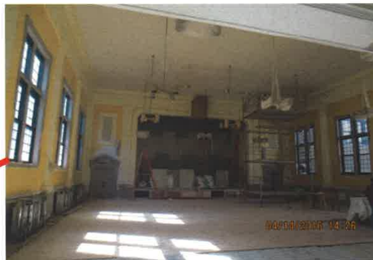
Auditorium Flooring Underlayment
